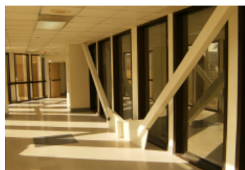
Bridge Seismic Bracing
